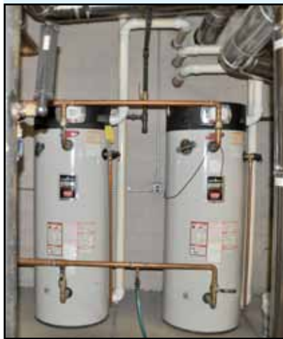
By upgrading the facility's equipment, Holy Spirit High School realized significant savings on energy use, service and fuel costs.
