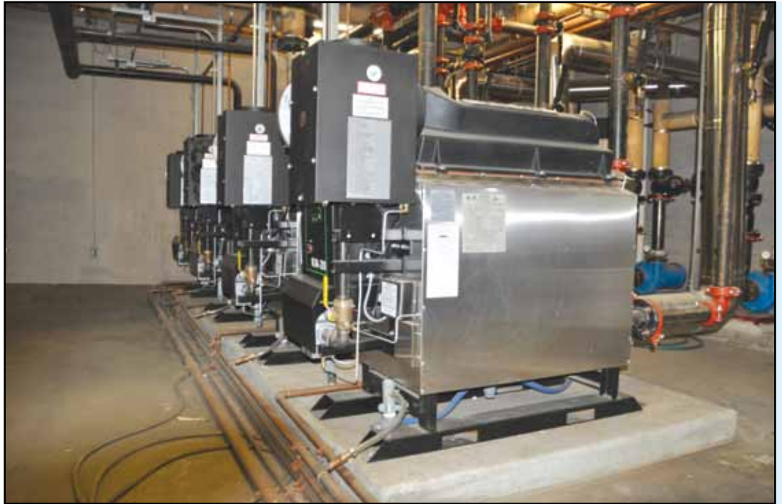
By design, high-efficiency modern natural gas boilers use 20%- 30% less energy than high mass oil burners.
